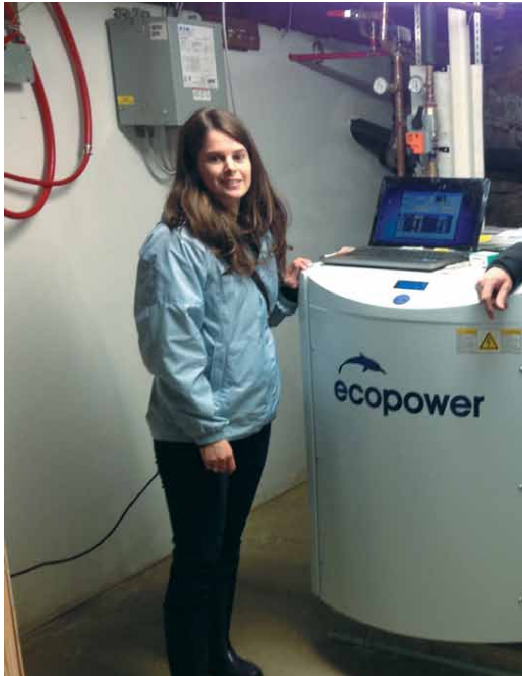
Ecopower Cogeneration Unit fuelled by Propane at Smugglers Cove Inn, Lunenburg, Nova Scotia
